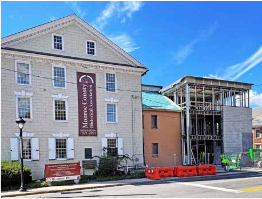
The Heritage Center addition to the Stroud Mansion is taking shape on 9th Street.
